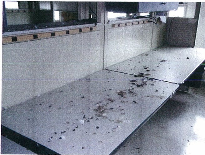
Photo 26: Bird droppings on upper floor of tower
