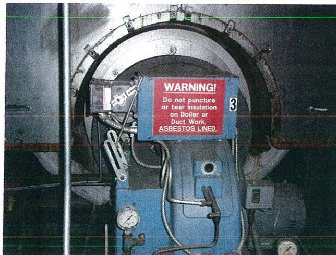
Photo 12: Boiler with asbestos labeling
