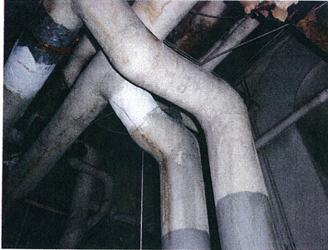
Photo 7. Mechanical room TSI assumed ACM
