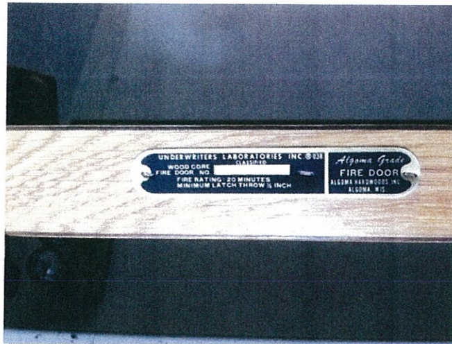
Photo 16: Fire door potential ACM
