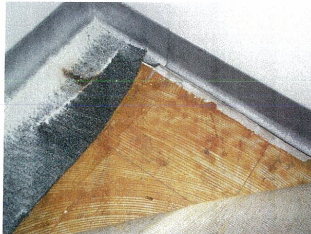
Photo 17: VFT beneath carpet
