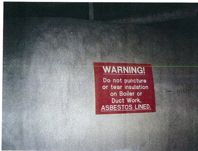
Photo 11: Boiler wrap with asbestos warning
