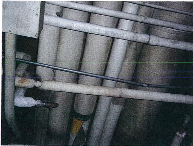
Photo 8. Mechanical room TSI assumed ACM
