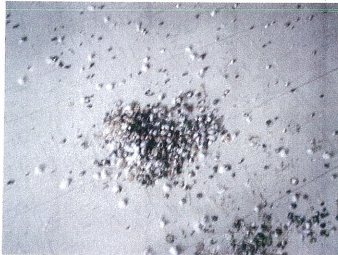
Photo 27: Bird droppings on upper floor of tower
