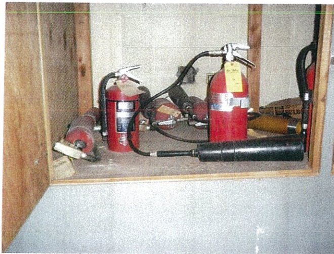
Photo 24: Compressed cylinders – fire extinguishers
