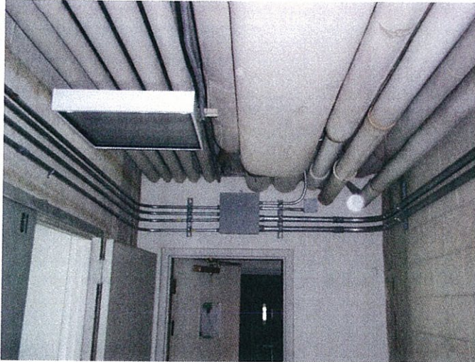
Photo 13: Hallway TSI assumed ACM
